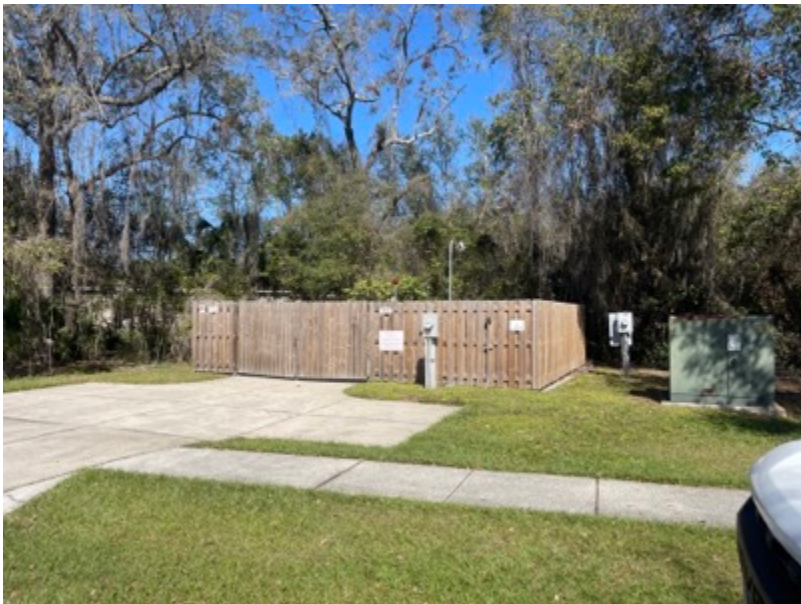
Facet View Pump Area Property Manager Pump area is being maintained and all conservation around has been pushed back
